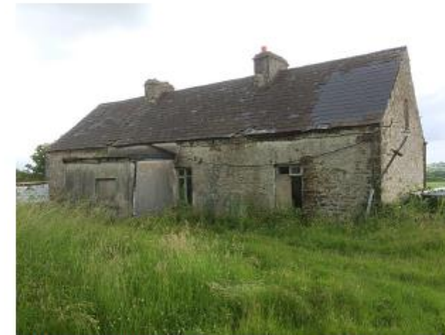
Image 4.1 An example of a derelict cottage (near Listowel) which were the most common site type within the survey area.
