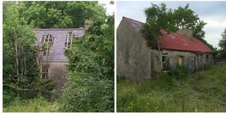
Image 4.2. Two story house near Listowel and cottage at Shrone East, a Category 2 and Category 3 site respectively.
